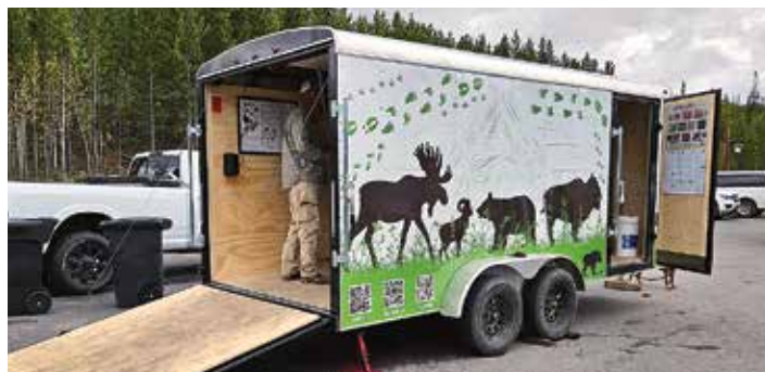
The wildlife education trailer under construction at the Spanish Peaks Mountain Club.
